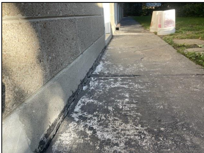
Improper slope or drainage
