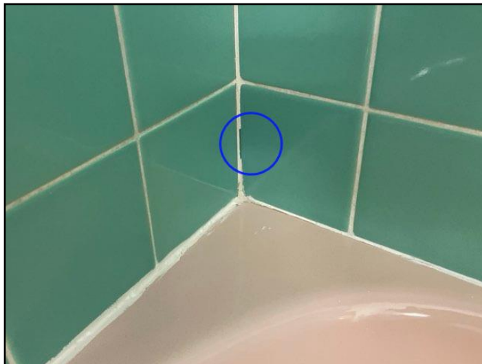
Caulking missing - second floor
