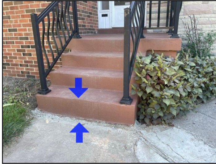
Stair rise too big or not uniform
