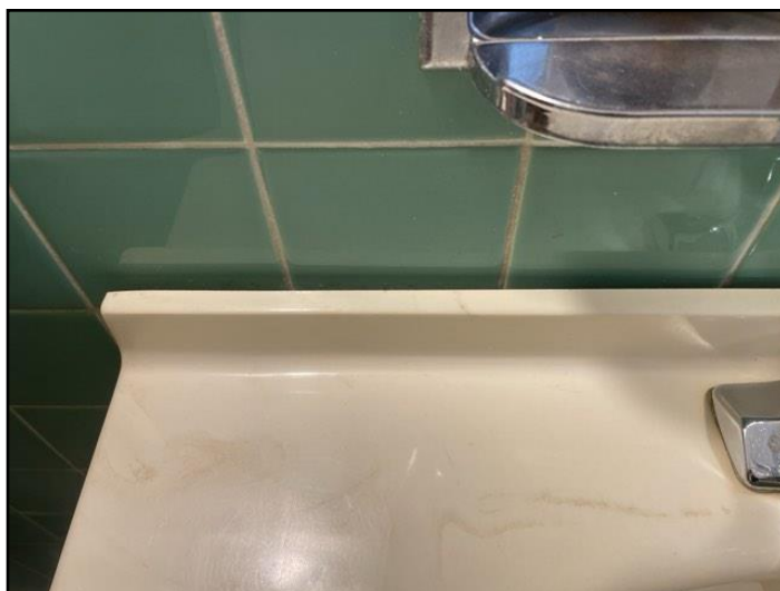
Caulking missing - second floor
