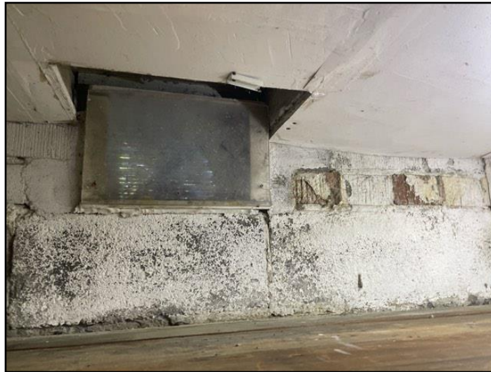
Vent(s) missing/not visible
