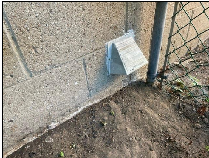
Too close to grade
