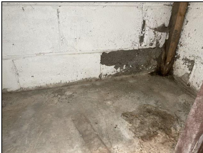
wood with moisture stains
