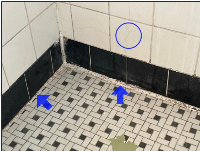
Caulking deteriorated-Crack tile - Basement
