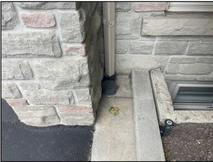
Discharge below grade
