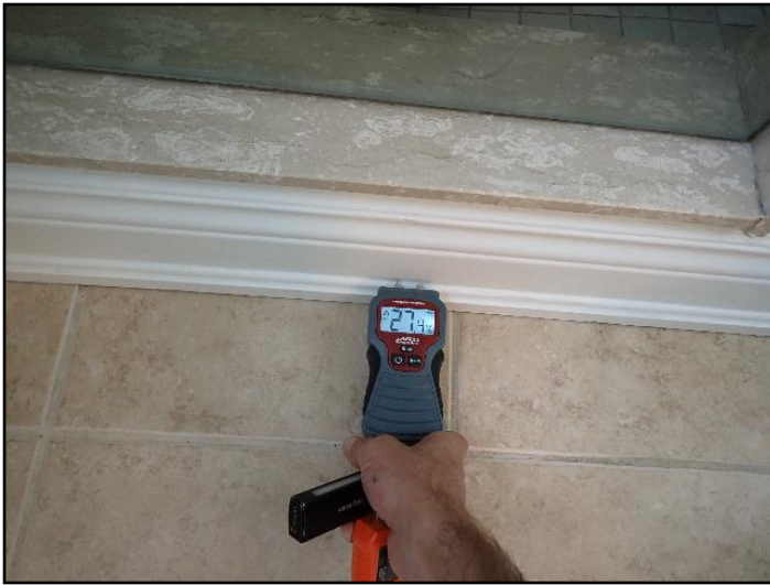
Elevated moisture noted on the trim below
