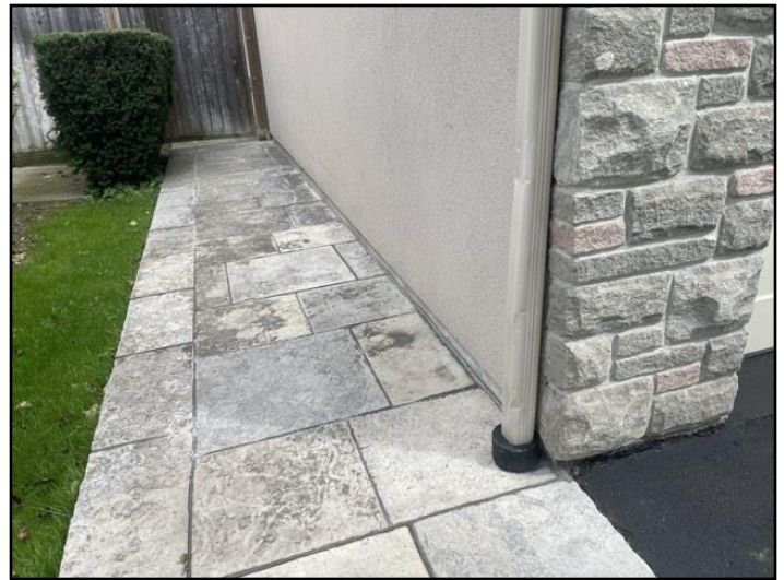
Discharge below grade
