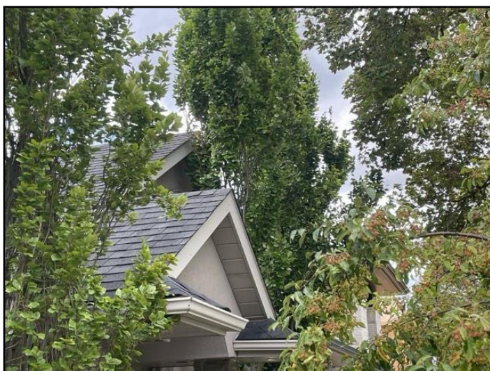
Tree branches touching roof
