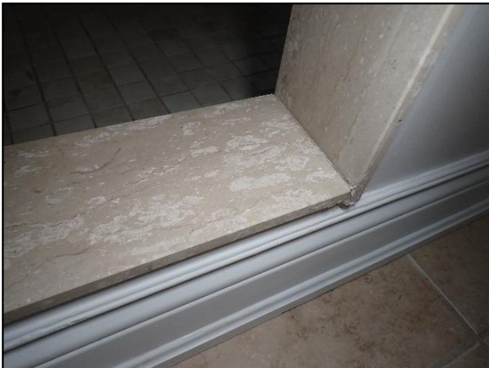
Caulking missing or deteriorated-Basement
