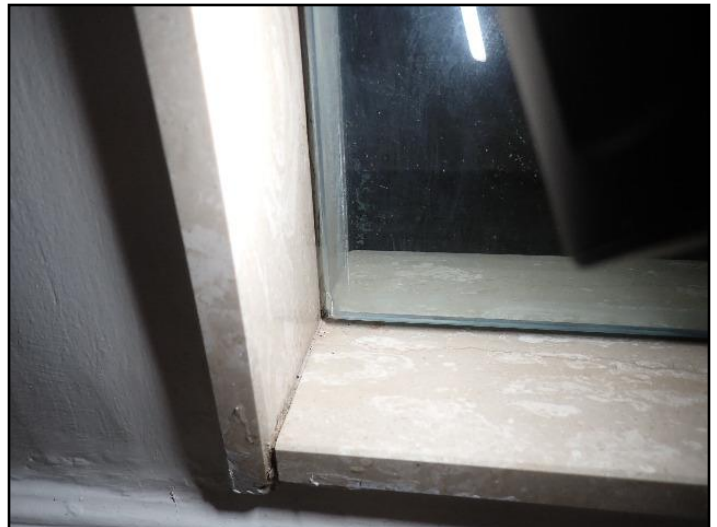
Caulking, missing or deteriorated-basement
