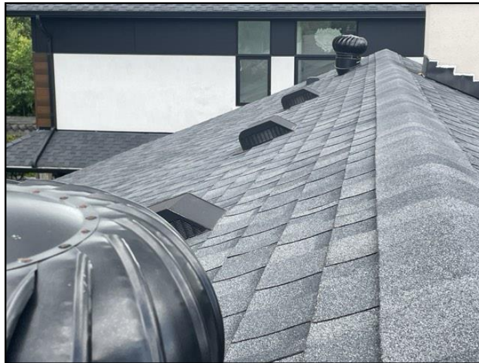
Roof vents (turbine type)
