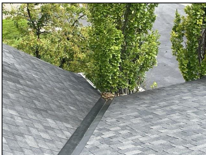
Tree branches touching roof
